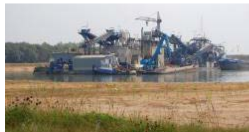
All inclusive Smals floating plant, extracting, processing and directly loading a customer's boat.
